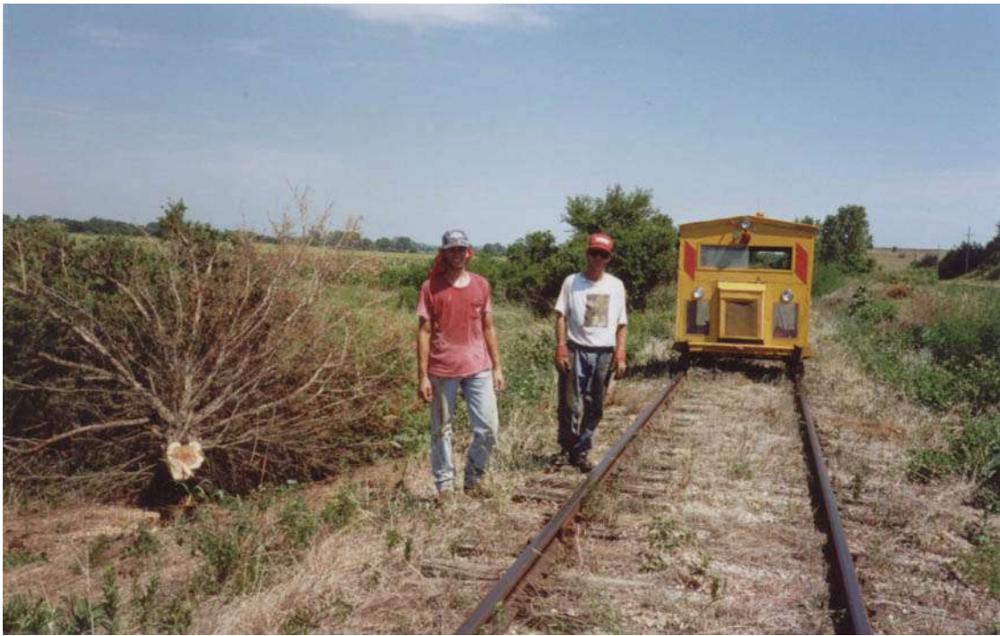
RAILSCENE: Working on the railroad: Employees Scott Egbers and Lawrence Addleman clearing the line of trees and brush, July 2002; temperatures in the 90's.
